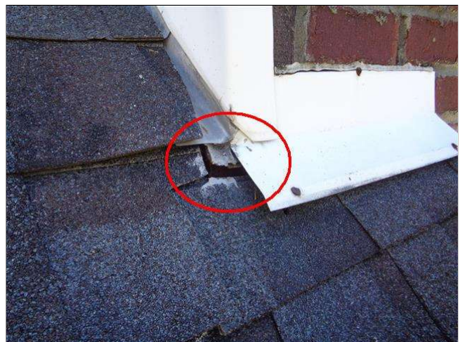
1.2 EXPOSED FLASHING Picture 2
