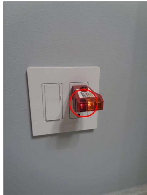
6.7.A ELECTRIC / GFCI Picture 1
