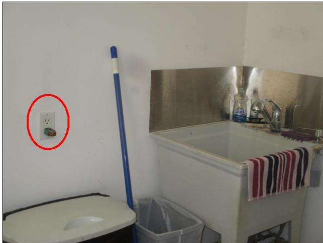
4.9 ELECTRIC / GFCI Picture 1
