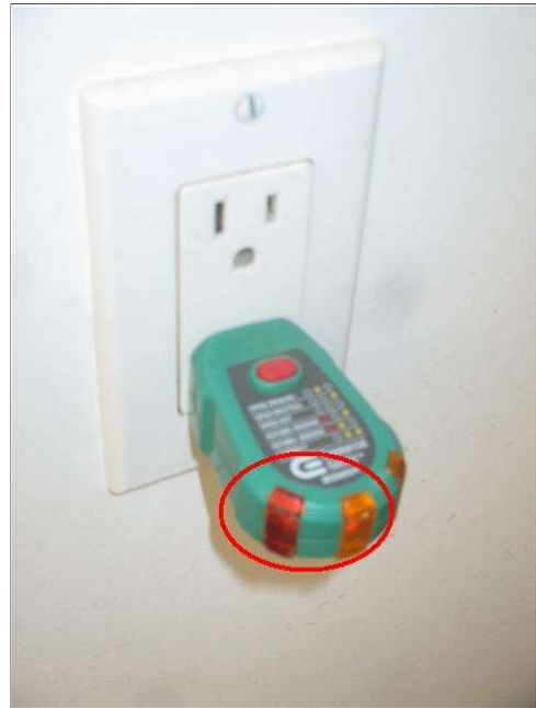
4.9 ELECTRIC / GFCI Picture 2
