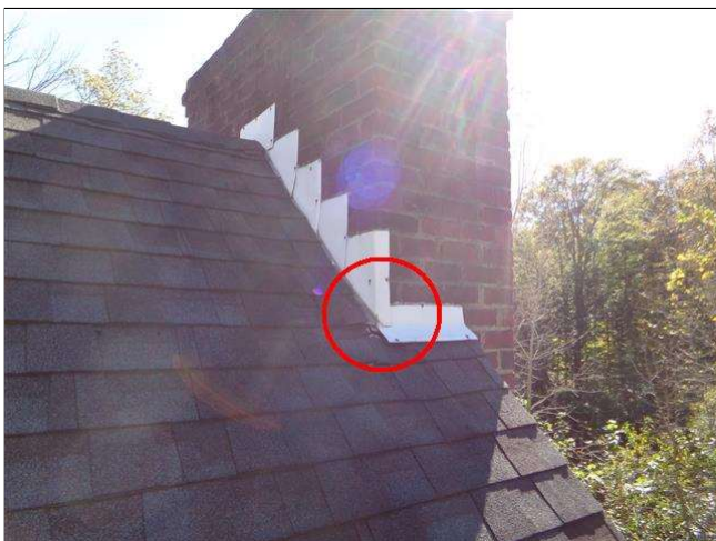
1.2 EXPOSED FLASHING Picture 1
