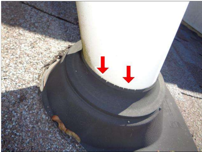
1.4 PLUMBING STACKS Picture 1
